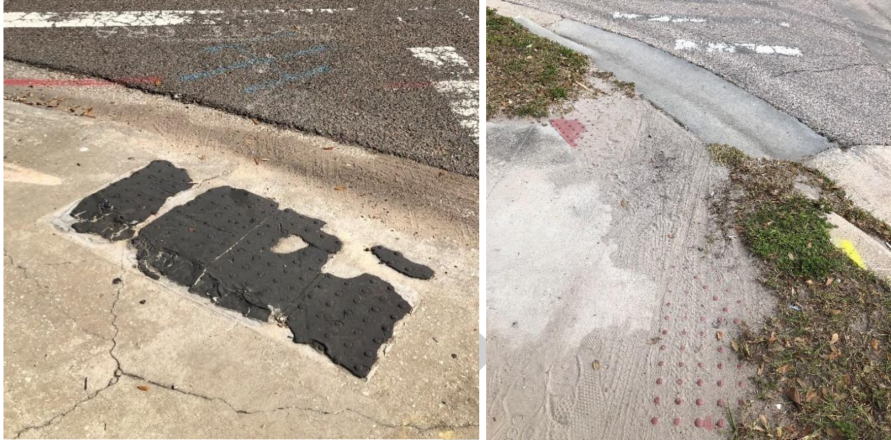
Figure 18: Worn Out/Obstructed Tactile Pads
