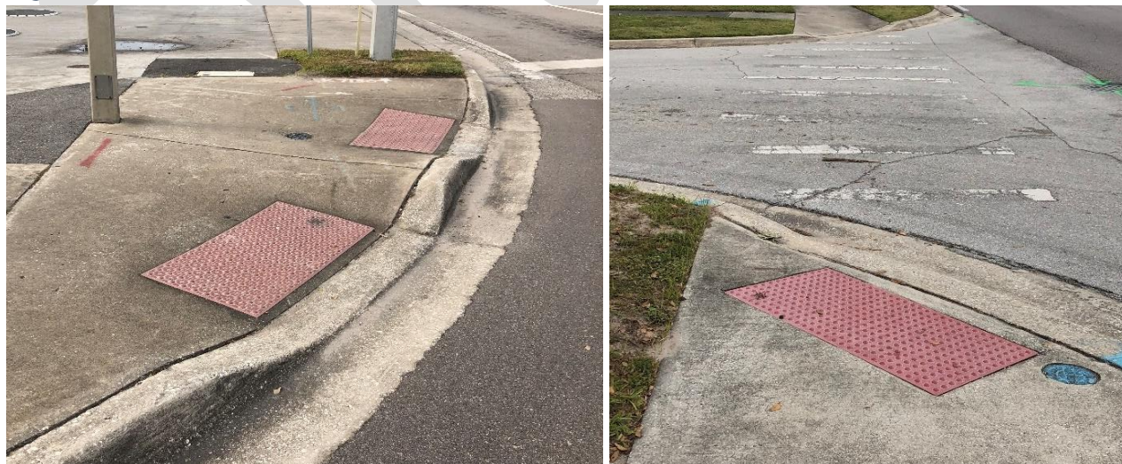
Figure 17: Improperly Installed Tactile Pads
